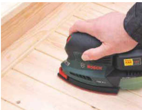
STEP 21. Fill nail holes and any defects. Sand all surfaces with 120 grit abrasive or finer, before dusting down
